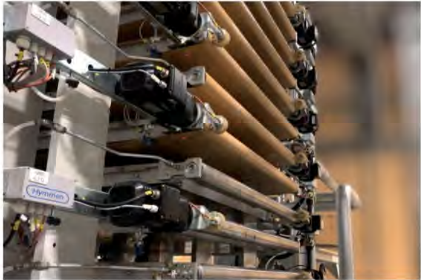
Hymmen plant components to produce engineered wood
